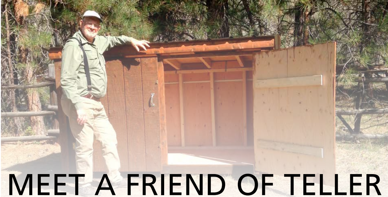
Ron Plakke spent 56 hours buying materials and constructing and staining the shed for Teller's new recycling program at Otto's Cabins. Many thanks to him and Teller Board Emeritus member Grant Parker, who helped with construction.
